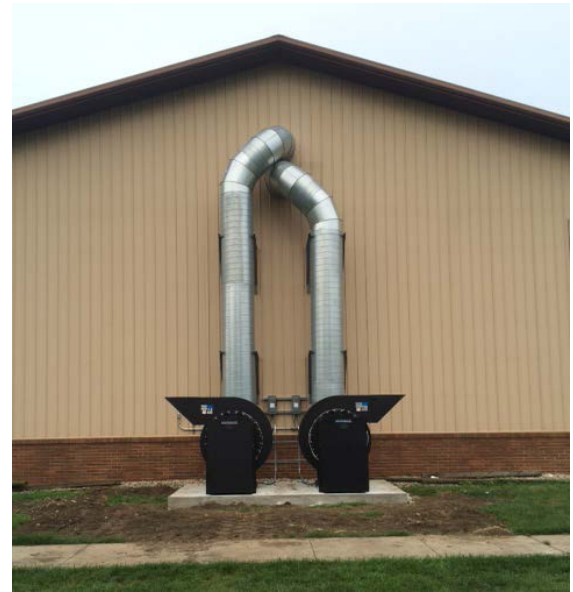
Ground Mounted MHA Blowers
